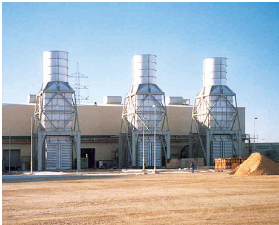
Gas turbine power plant in the Libyan town of Zawia (© Bilfinger Construction GmbH)
